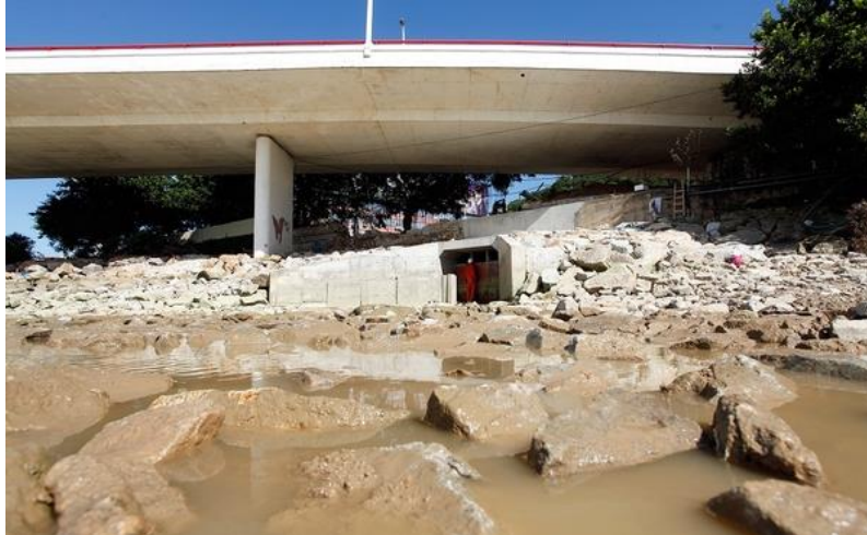
Figure 5 Building a new drainage system in the Taipa Hill to bypass the rainwater.
